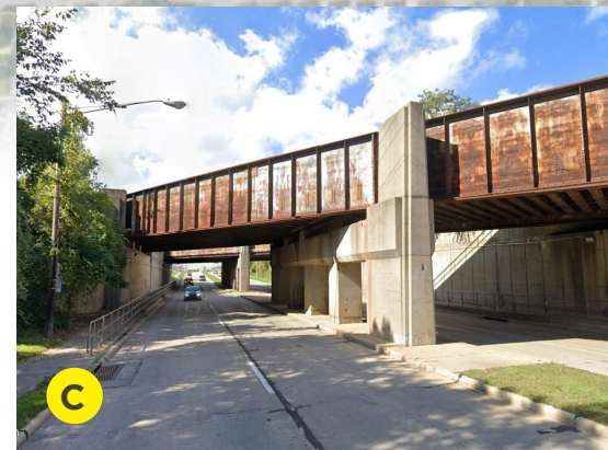
C The Railroad underpass has existing sidewalks, but is poorly lit and creates a perceived barrier along Vine St, especially to pedestrians.
